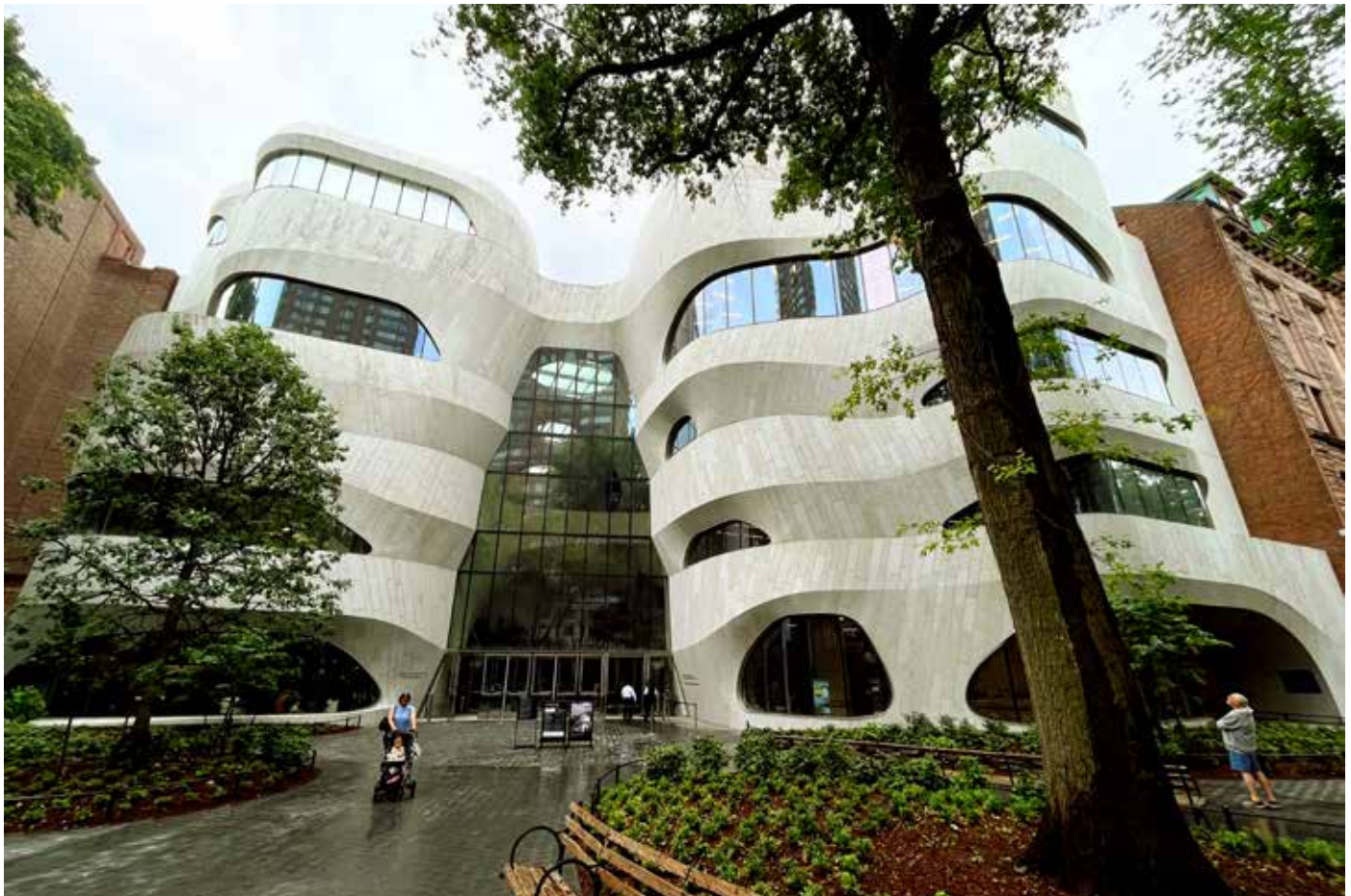
Above and Opposite: COST of Wisconsin used specialized shotcrete and rebar techniques to construct the interior and exterior walls of the Gilder Center at AMNH. All photos are courtesy of COST of Wisconsin
